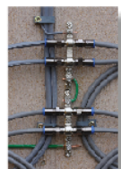
Multiple Ground Blocks
